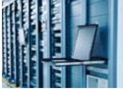
Control Center/Data Center
